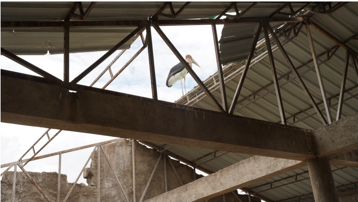
The missing roof panels
